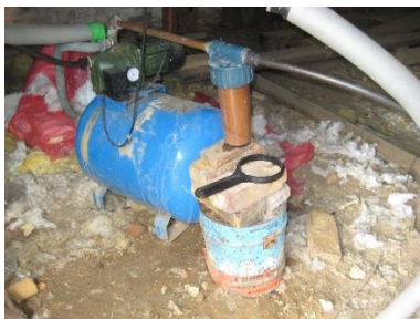
Water supply with inadequate filtration system
